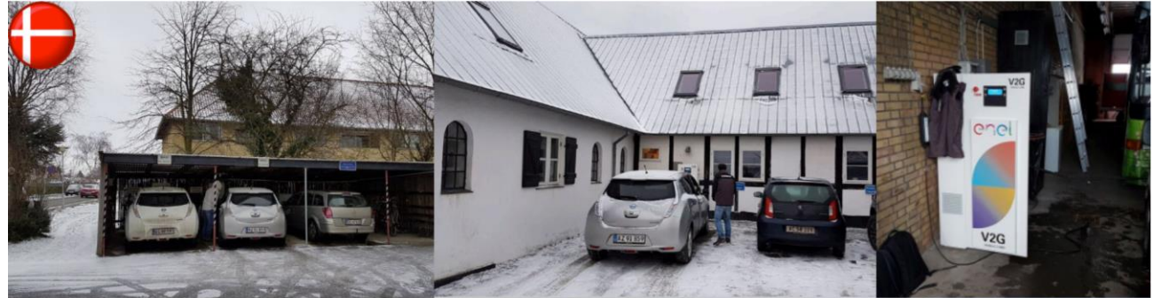
DENMARK V2G installations
