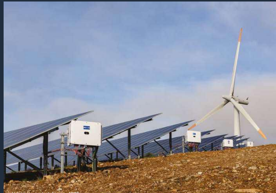
Hybrid power plant. Source: EDPR
