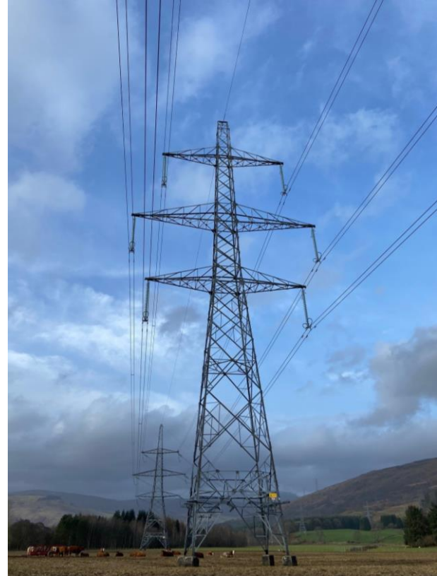
Beaully-Denny overhead line
